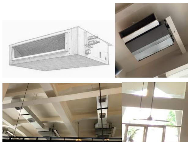
Fig. 8. HVAC and fans units in restaurant.
